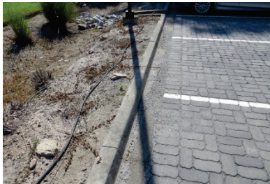
6 Unstable drainage area
