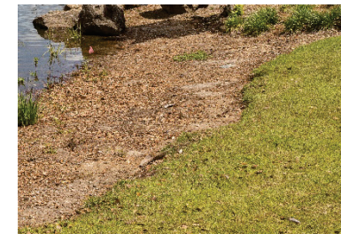
21 Erosion, plant, mulch
