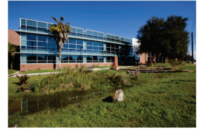
10 Presence of ponding
