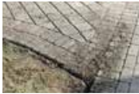
6 Unstable drainage area
