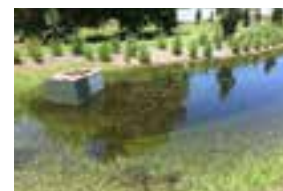
13 Presence of ponding
